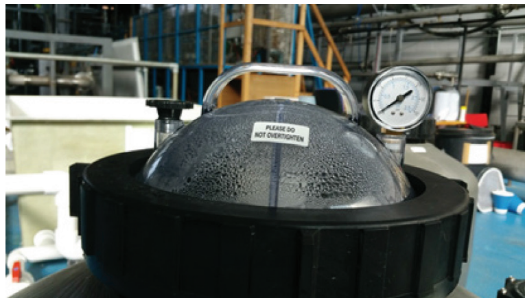
Pressure gauge mounted on top of the filtration vessel
